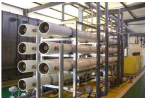
渗沥液处理设备 Leachate treatment equipment
