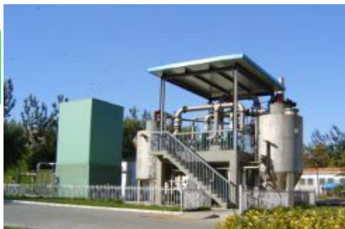
沼气发电设备 Biogas generating equipment
