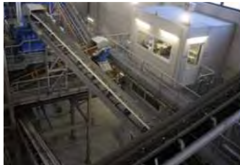
Glass sorting plant Asti Capacity: 180 kt/y
