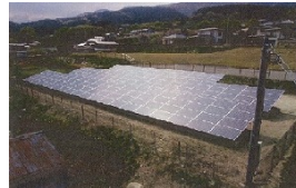
Photovoltaic power generation business (in Iida City)
