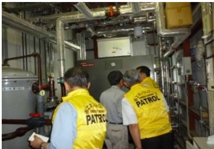
Shinshu Energy-saving Patrol Team Energy-saving diagnoses of equipment and facilities conducted by volunteers.
